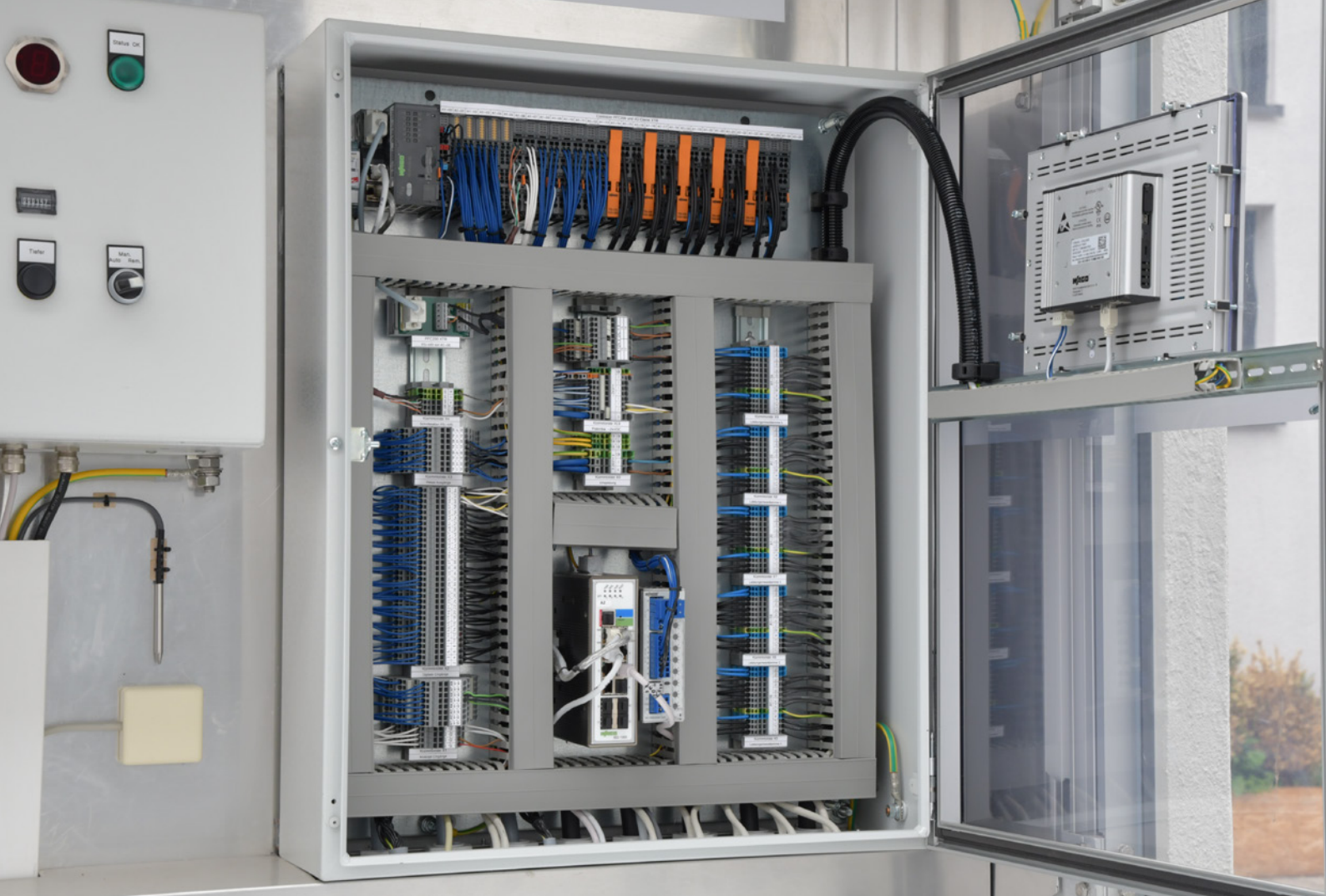
Rail-mount terminal blocks in use in a substation
